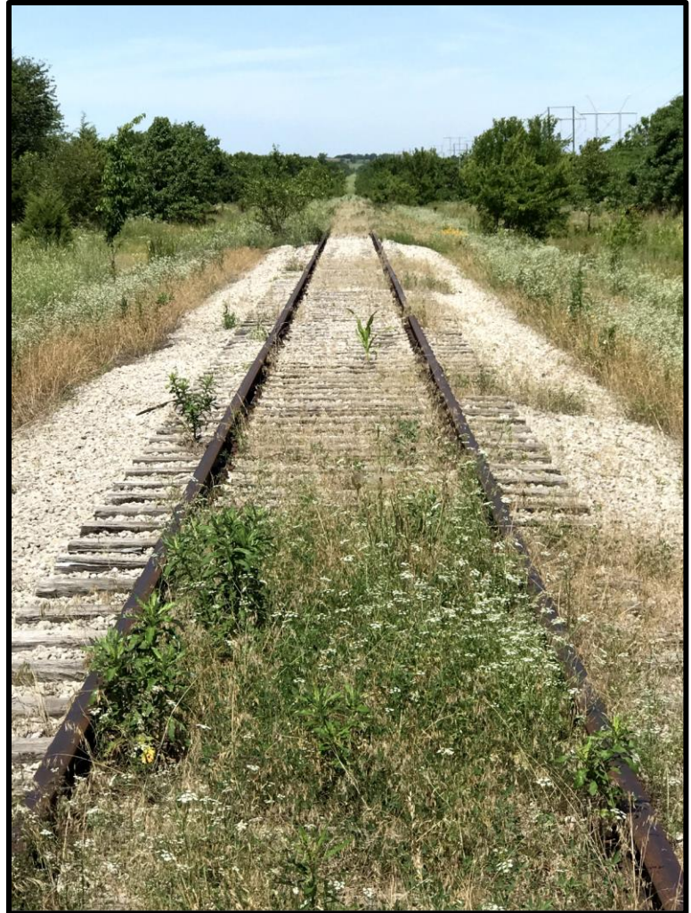
Figure 1: Existing spur track unused and in disrepair.
